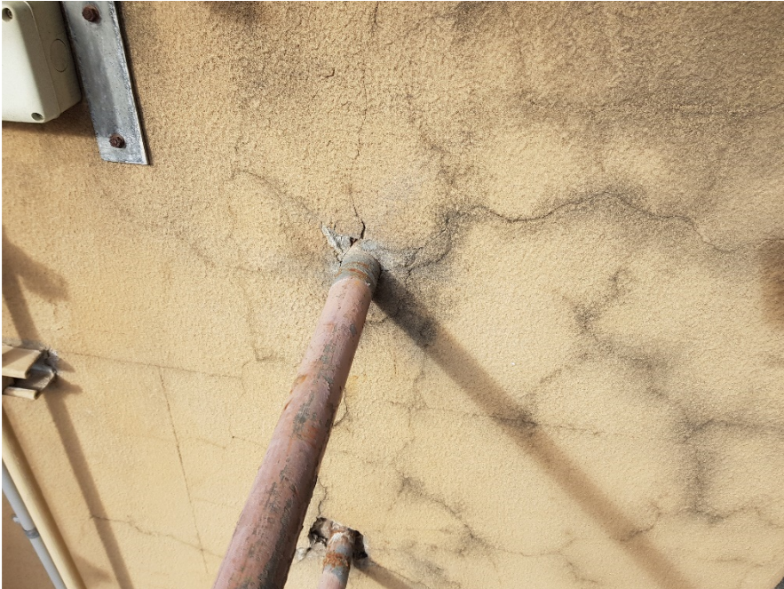
Figure 9: Cracking Around Embedded Railing
