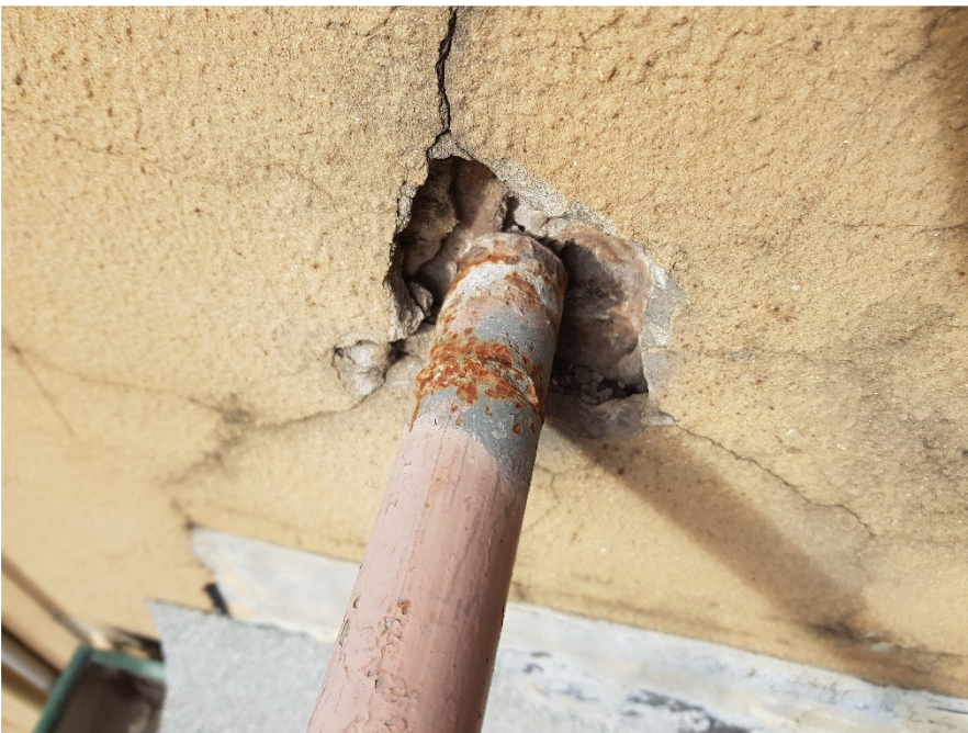
Figure 8: Original Railing Broken Off from Wall
