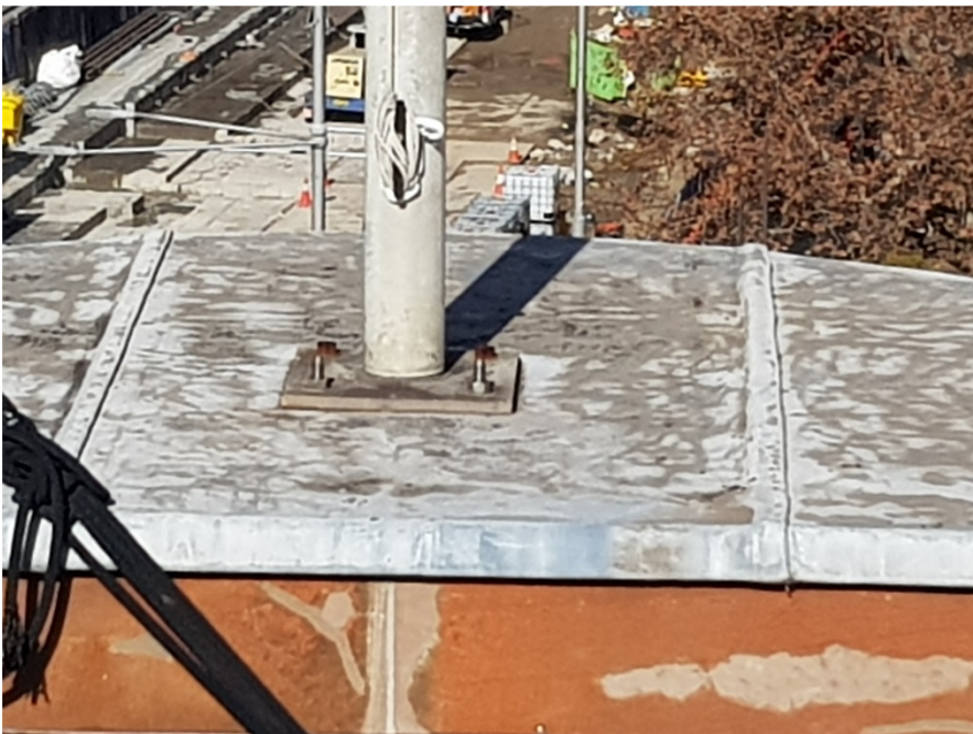
Figure 4: Corroded Flag Pole Connections South End
