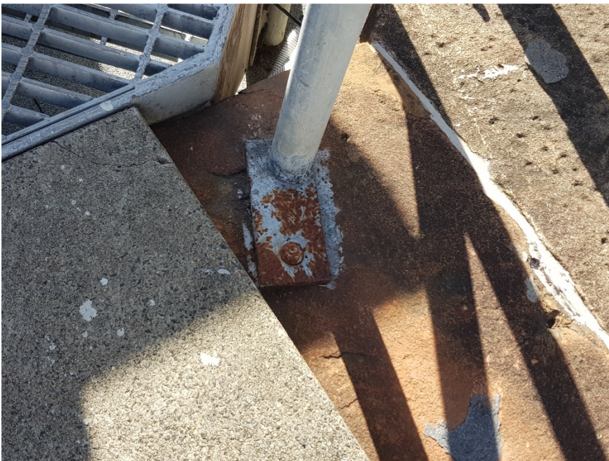
Figure 10: Corroded Connection of Access Structure South End
