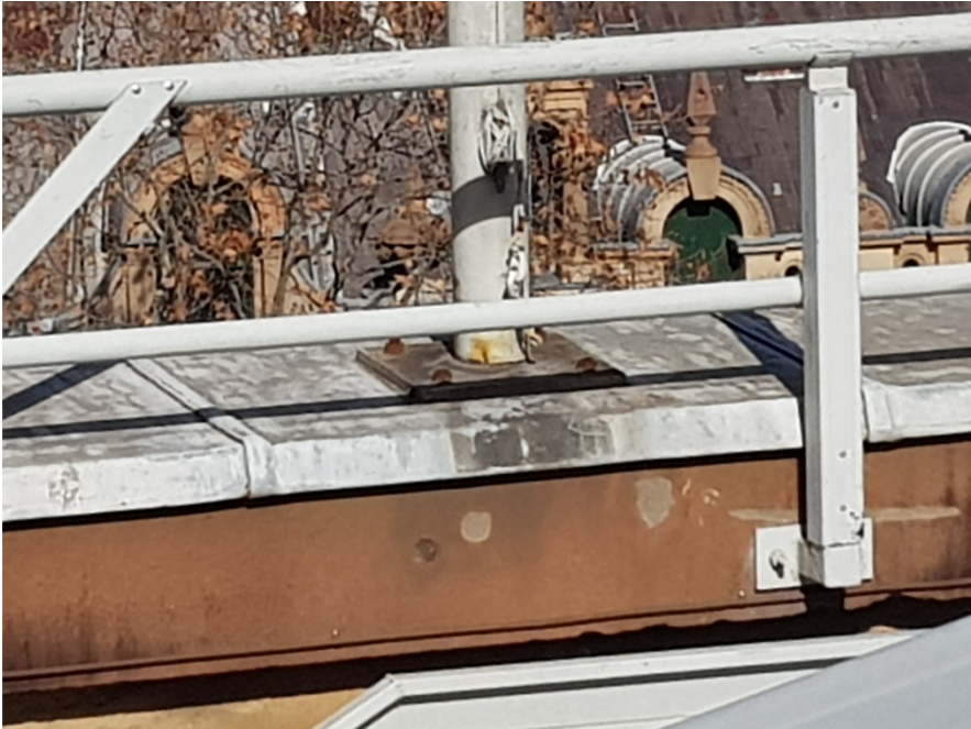
Figure 5: Corroded Flag Pole Connections South End
